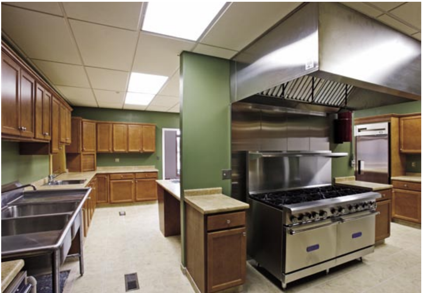
The commercial kitchen designed and built for Calvary Bible Church by Bossart Builders features a Royal commercial stove and ovens, two True side-by-side refrigerators, maple Homecrest kitchen cabinets supplied by building partner Barden Homes, double commercial stainless sinks, two microwaves, two convection ovens, one freezer and a 22-foot-long walk-in pantry.
