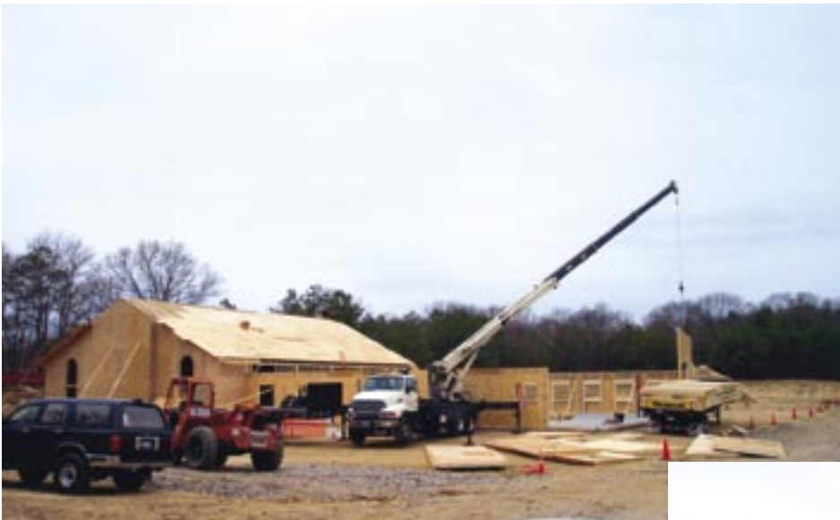
Left: The Rock of Salvation Church, being erected with the Barden pre-manufactured panel and truss system, is located in Islip, Long Island.
