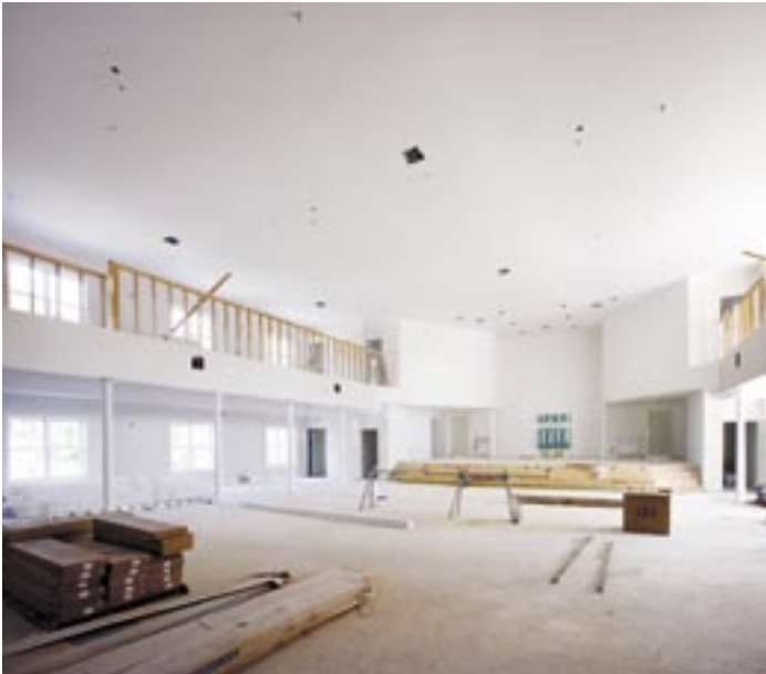
Christian Community Chapel in Hillsboro is an independent Bible-based mission currently under construction by Bossart Builders. Pictured here is the church sanctuary, altar and balcony for additional parishioners' seating.
